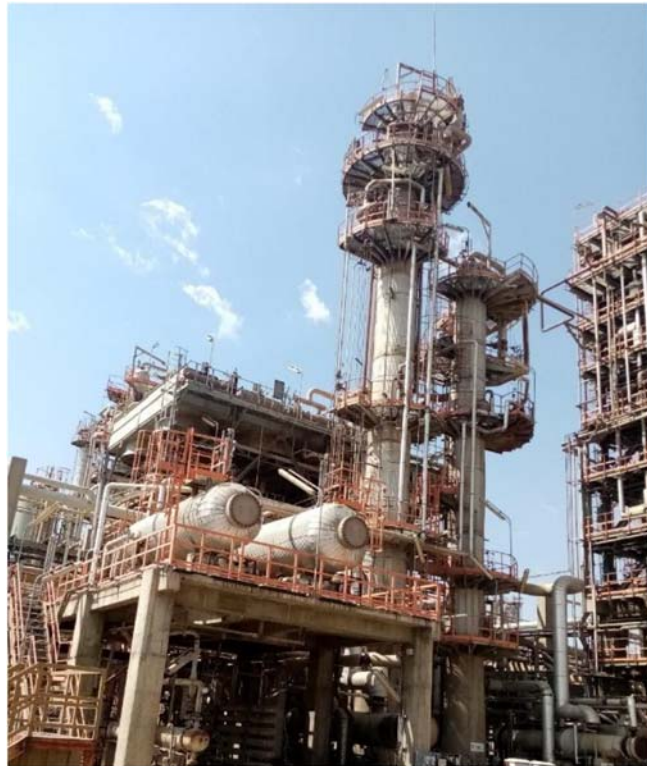
Figure 7.1 A part of a petrochemical plant including absorption towers and horizontal drums.
