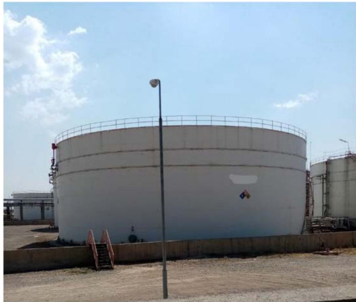
Figure 7.4 An external floating roof tank.
