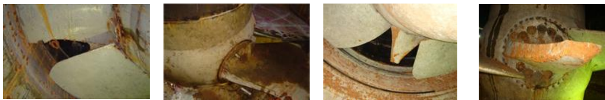
Figure 1. Damaged runner blades.
