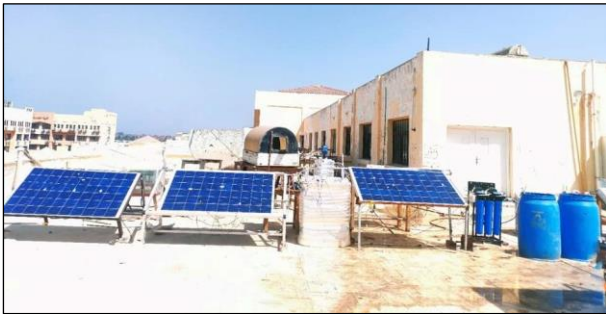
Figure 13. Solar-powered reverse osmosis desalination plant [63]
