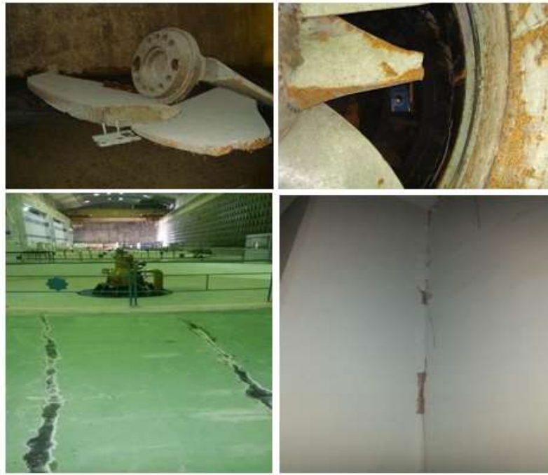
Figure 4: Runner blade damage (top), and structural cracks in Haditha HPP (bottom) [13].
