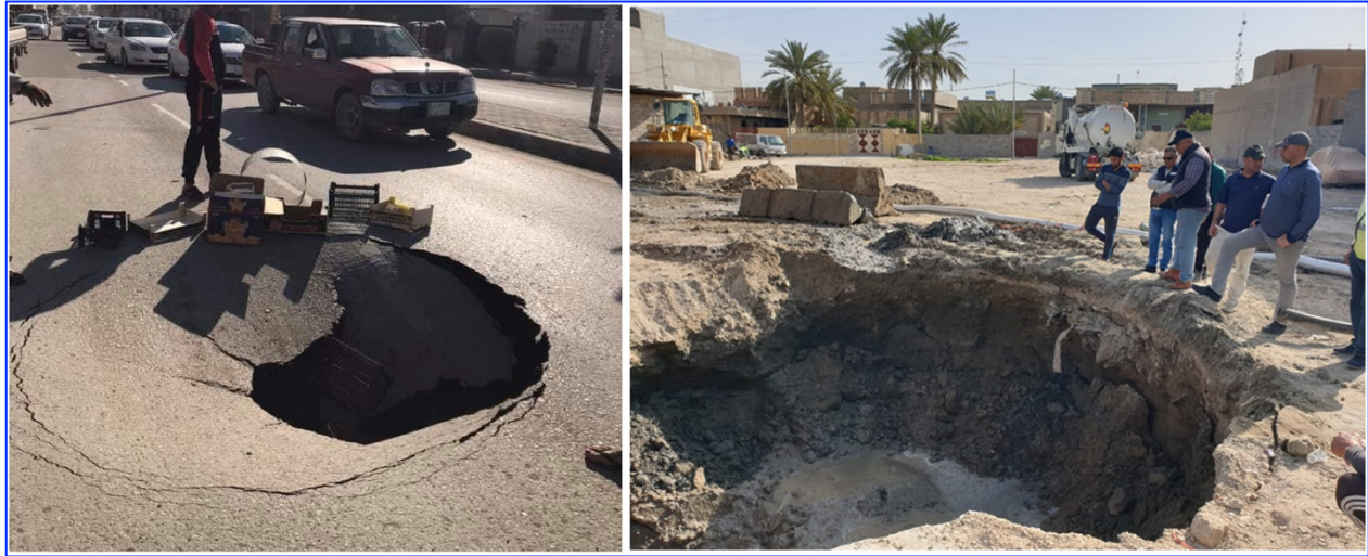
Fig. 3. The subsidence of a hole in Omar bin Abdul Aziz Street within the city of Ramadi
