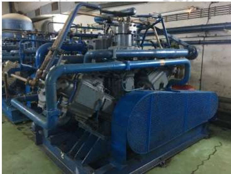
Figure 1. The compressed air system in Haditha HPP (courtesy Haditha HPP-MOE Iraq).
