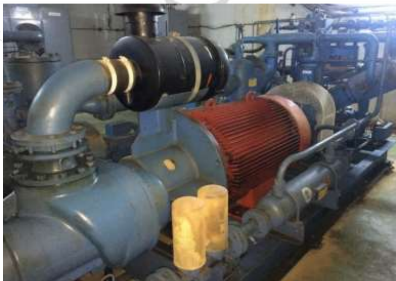
Figure 2. The compressor electrical motor used in Haditha HPP(courtesy Haditha HPP-MOE Iraq).
