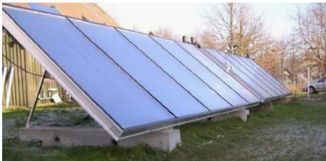
Fig. 1. Photograph of the flat plate solar collector (Kong et al. [33]).
