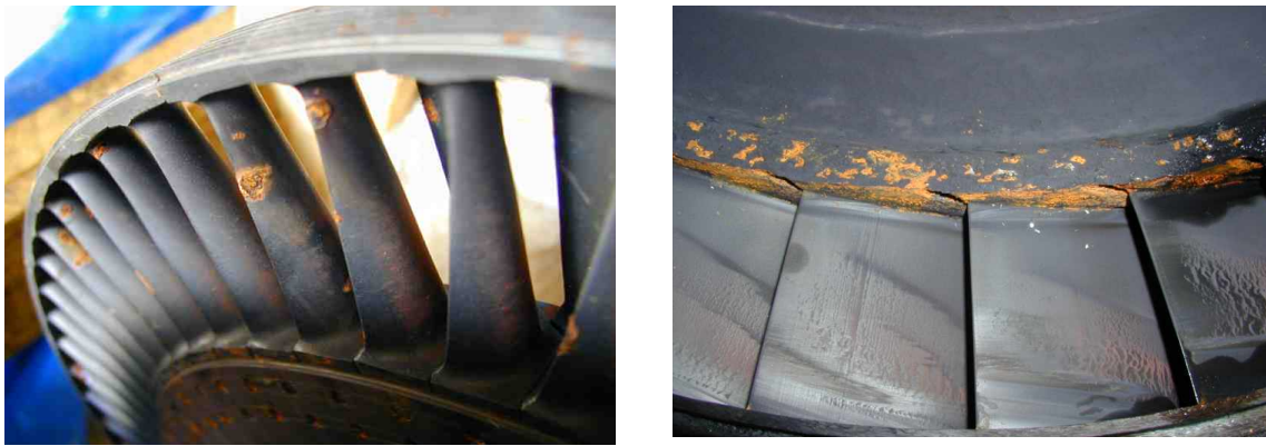
Figure 6: Erosion and pitting of steam turbine blades [10]
