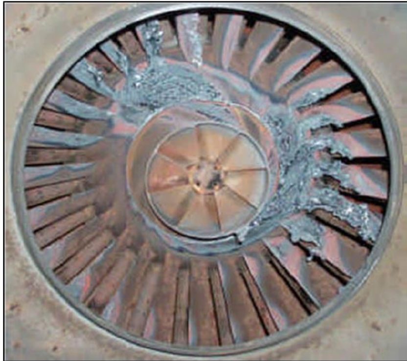
Fig.1 2 System hardware damages due to flashback.
