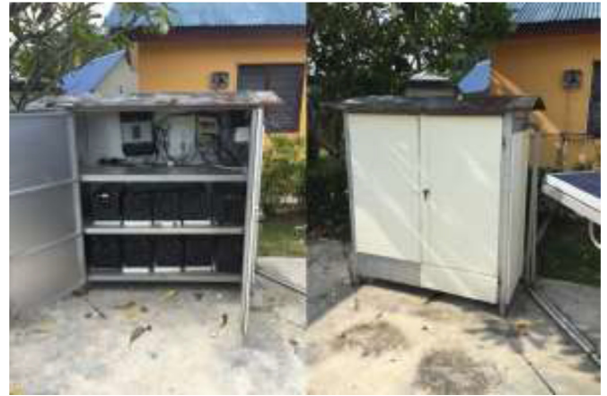
Fig. 21. Photo of battery bank room.
